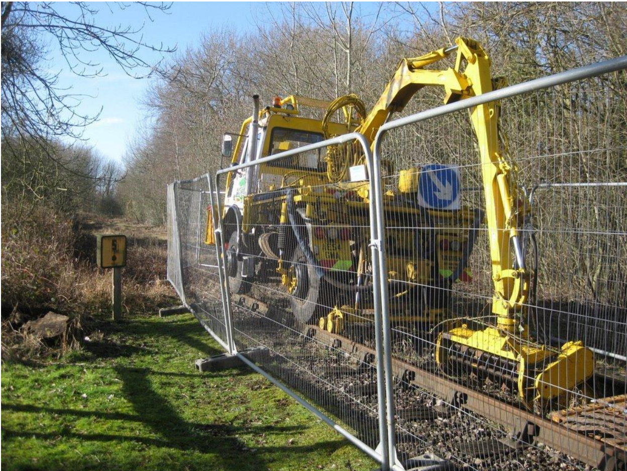
Above: Track clearing machine working near Swanbourne (26 miles west of Bedford) (John E Levin)
