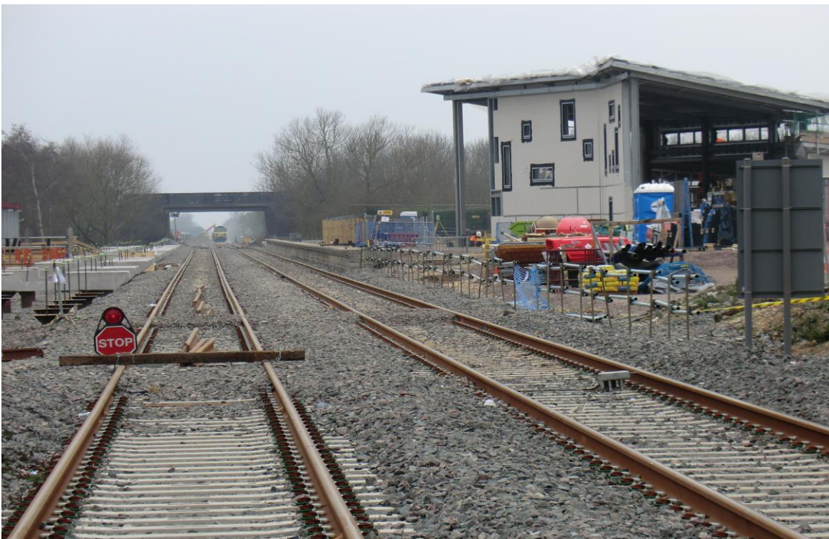
Above – centre & right: new track and station building at Bicester; left: new platform under construction. (John Elvin)
